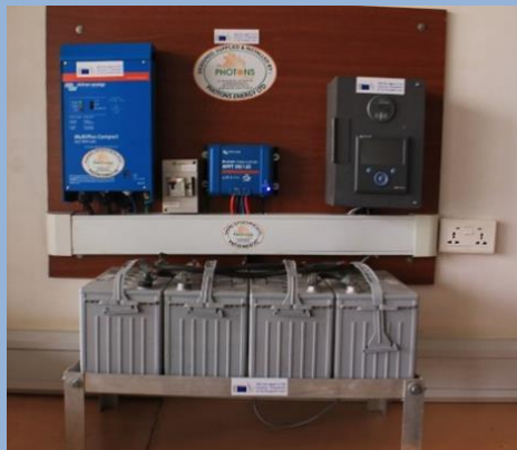
Medium PV System
